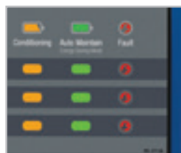
Battery fault detection LEDs
